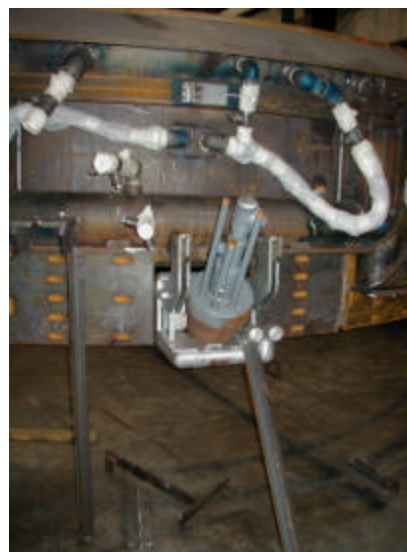
(b) EBT installation (typical)
