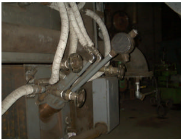
(a) Side-wall installation at JYXS
