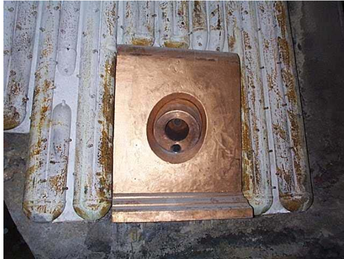
Fig 5 : PYREJET™ and its associated copper panel
